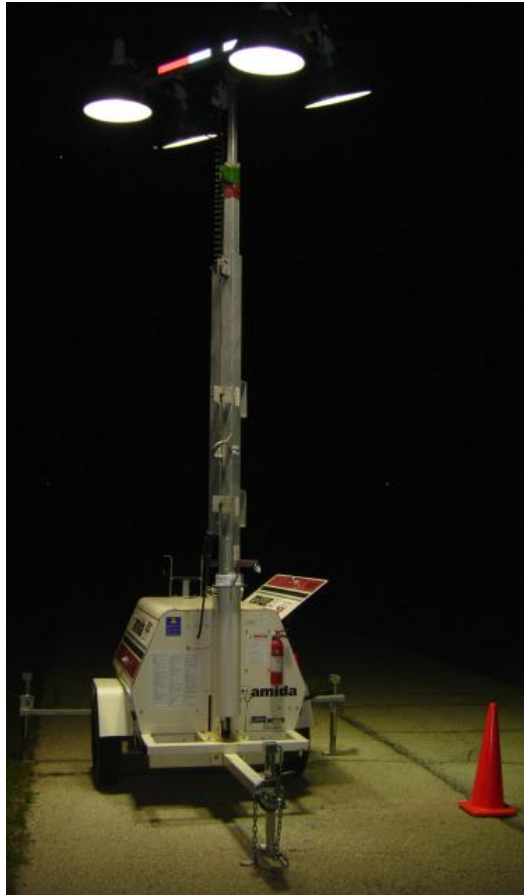
Figure 4.48 One Light Tower Arrangement
